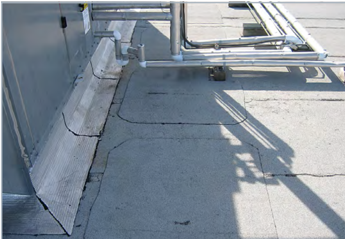
1. Repair and replace any deteriorated areas with LIKE MATERIALS to make WATERTIGHT.
