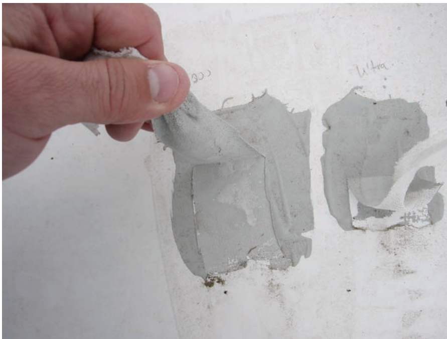
A field adhesion test, demonstrated in the photo, will help ensure a successful coating application.
