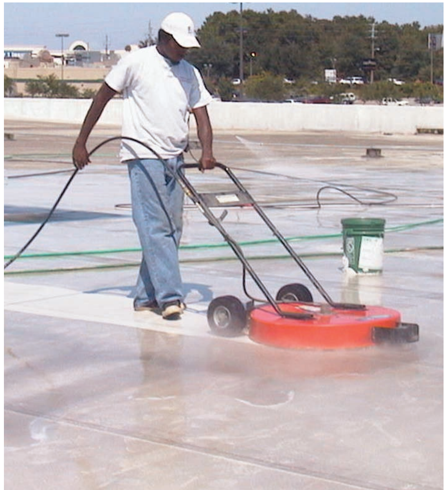
For proper adhesion, a roof substrate must be cleaned and prepared satisfactorily; most roof surfaces are best cleaned by power washing.
