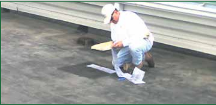
Address all problem areas. Repair with like materials.
